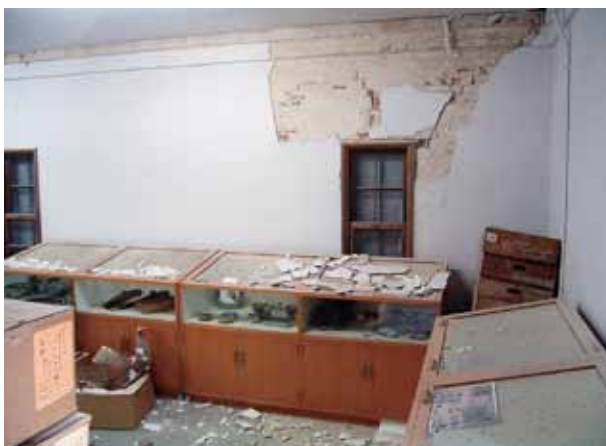
3階内壁の漆喰が崩落
